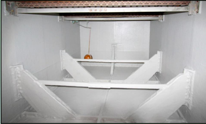
Water Tank GRP Lining
